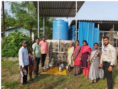
Drinking Water Facility Sand Filter At – Pale khurdi Village Roha - Raigad
